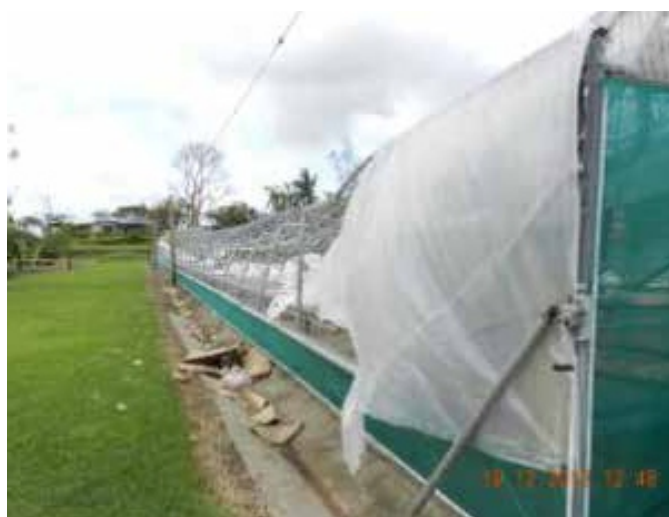
British American Tobacco nursery in Nadi suffered significant damage to the plastic covering and steel frames as a result of TC Evan. Clearly, 'disaster resilient' nursery design practices need to be incorporated into any agribusiness operating in cyclone prone countries such as Fiji.
